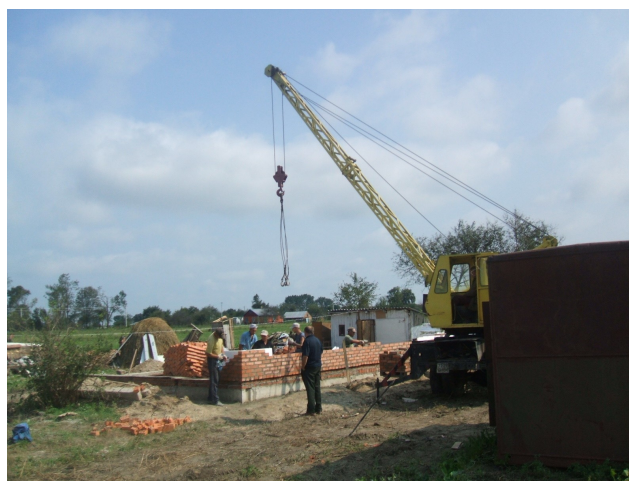
New houses were built for people who lost their property as a result of the storms
