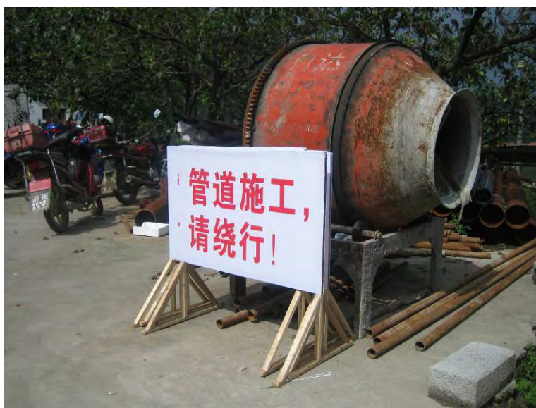
Onsite safety signs in the water treatment plant. Photo: IFRC
