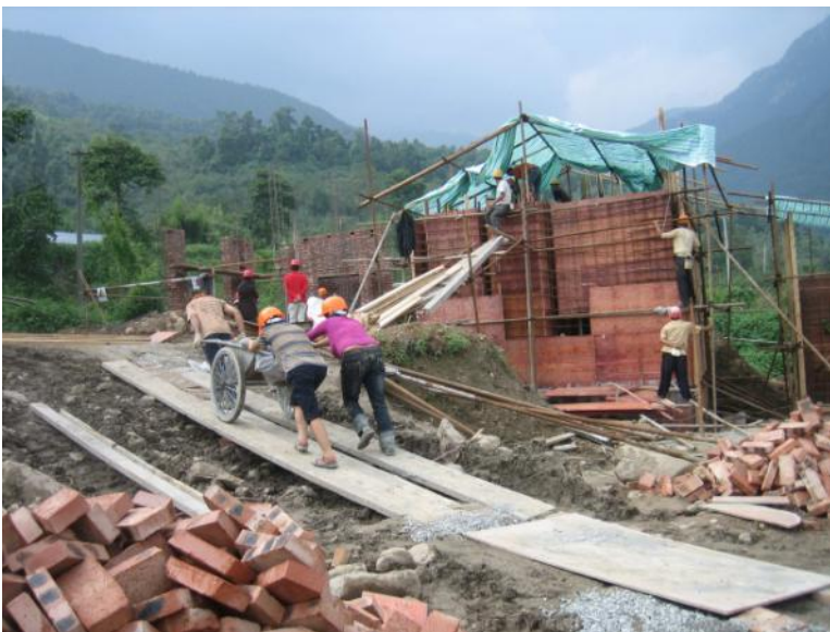
Sedimentation Tank and Filter Tank Construction at the water treatment plant site. Photo by IFRC
