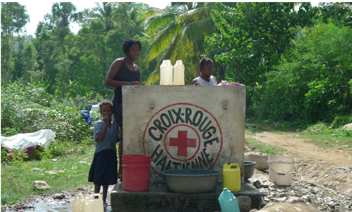
15,000 people have access to safe drinking water in Peredo (Sud-Est) through the rehabilitation of the clean water source and the implementation of a secondary pipe system.
