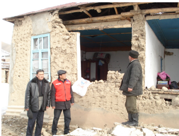
One of the houses severely damaged by the earthquake in Osh. Source: Kyrgyzstan Red Crescent, Osh branch
