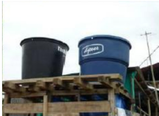
Water tanks were installed in homes of affected families. Source: Colombian Red Cross Society.
