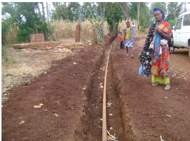
Trench excavation as part of the water and sanitation project in East Hararghe funded by British RC through this Appeal. Source: ERCS
