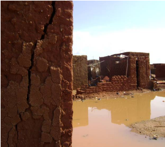
Thousands of homes either damaged or destroyed
