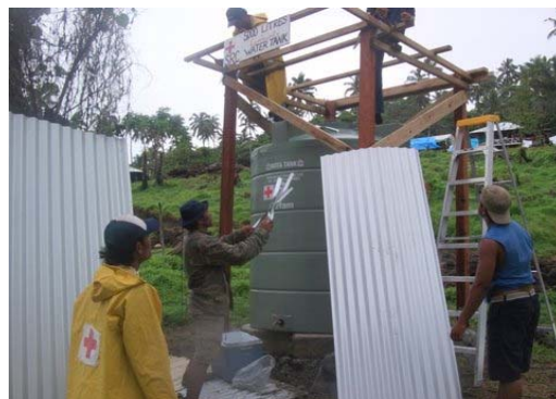
SRCS volunteers assist in constructing rainwater collection system in Lalomanu. Photo credit: International Federation/Victoria Fray.
