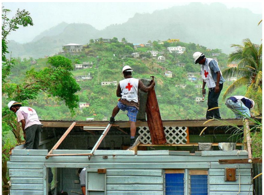
The Saint Vincent and the Grenadines Red Cross, with the support from ECHO, conducted a roofing workshop from 16 to 23 November with volunteers and government officials as participants. Source: SVGRC
