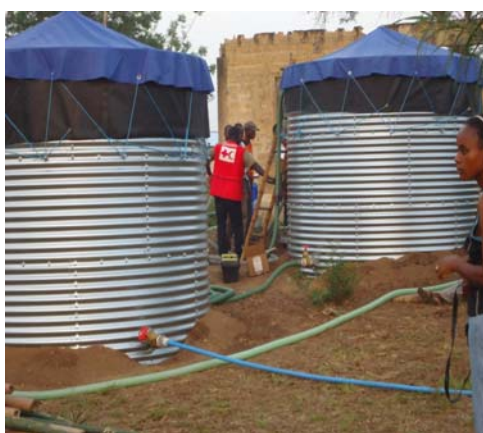
Water supply facility (Kit 5) installed by LNRCS trained volunteers and staff at Bortuo in Liberia. IFRC.
