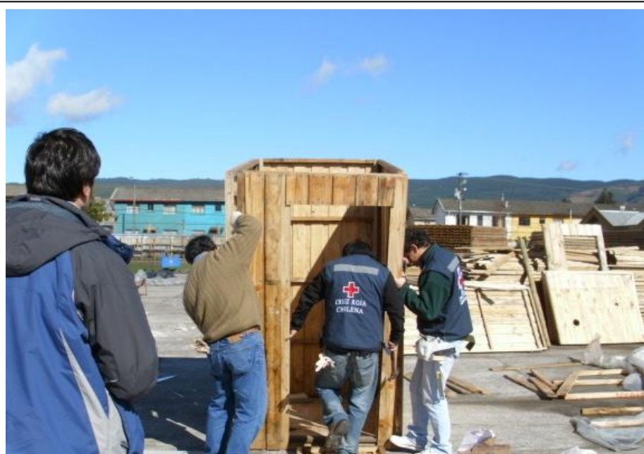
Chilean Red Cross volunteers, together with municipal work functionaries and village inhabitants, install one-family sanitary units. Source: Chilean Red Cross
