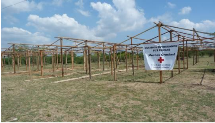
Construction of transitional shelters in Candelaria, Atlántico department that will benefit 100 families. Source: CRCS
