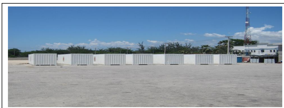
TMSUs in Barbancourt warehouse (Port-au-Prince)
