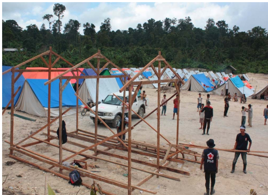
Palang Merah Indonesia volunteers are constructing shelters on a site on South Pagai Island. Palang Merah Indonesia has provided 516 families with temporary shelters before the end of this year. Photo credit: Palang Merah Indonesia.
