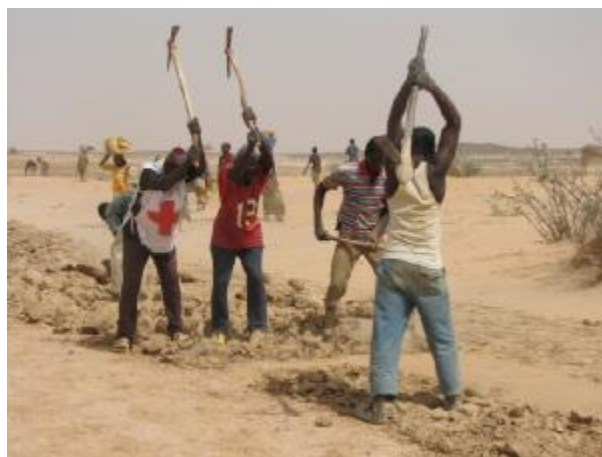
Beneficiaries rehabilitate land at Cash for work project site, Tahoua, Niger/ April 2010
