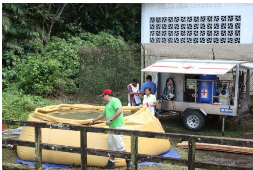
Volunteers from the Red Cross Society of Panama (RCSP) install the mobile water treatment plant in Portobello. Source: RCSP
