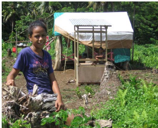
A household latrine under construction using materials donated by the Samoa Red Cross Society Photo credit: IFRC
