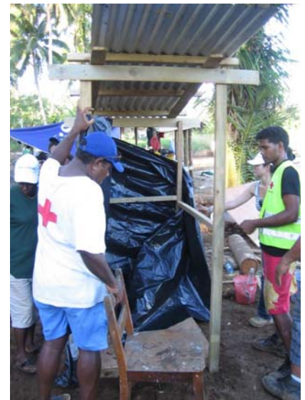
Participants constructing a latrine during the Water and Sanitation Emergency Response Training Photo credit: IFRC
