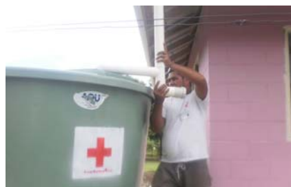
SRCS volunteer completes the final stage of installing a rainwater harvesting tank in November 2010 in Manono Uta village. This stage involves connecting the first flush component to clear up any foliage or matter in the water flow. Photo by SRCS.
