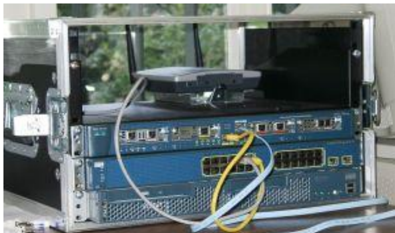
Prototype components mounted in frame. Note wireless access point.
