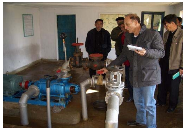
The assessment team visits the water and sanitation facilities in Hanumul-dong, Taedong county of South Phyongan province just before the handover.
