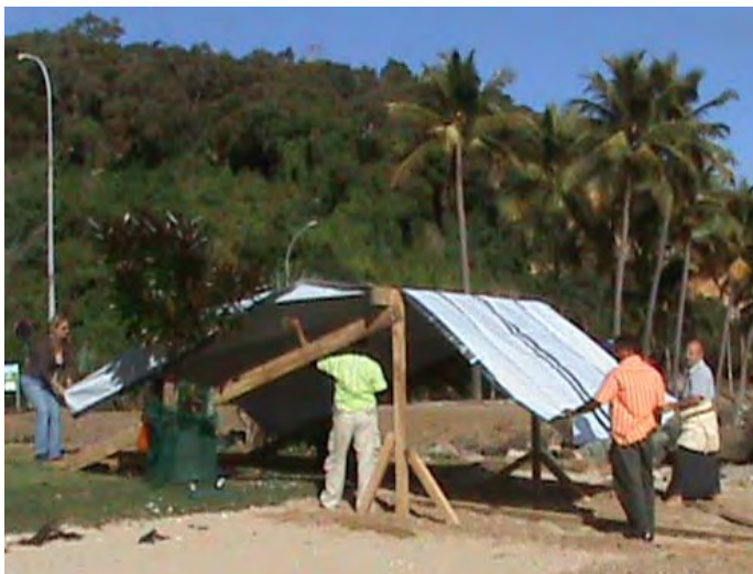
The disaster management forum organized in New Caledonia in June 2008 included a session on shelter, where participants were invited to exchange cultural perceptions of shelter and were provided with a better understanding of adequate shelter in an emergency context. This was followed by the opportunity to gain hands on experience using a basic shelter kit to construct their own shelters. International Federation.
