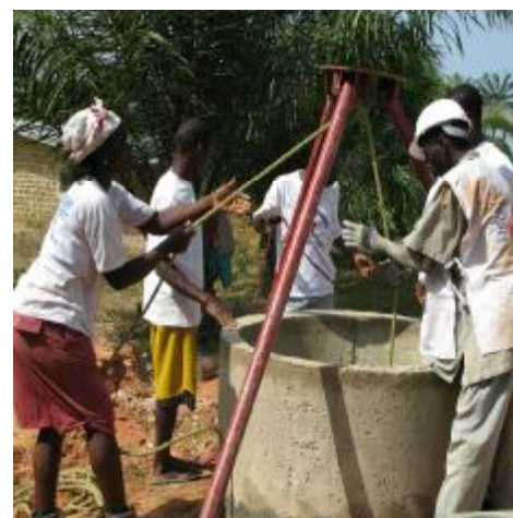
The water and sanitation projects of the LNRCS aim at contributing to reducing the outbreak of diseases in the rural communities in Liberia/ LRRCS
