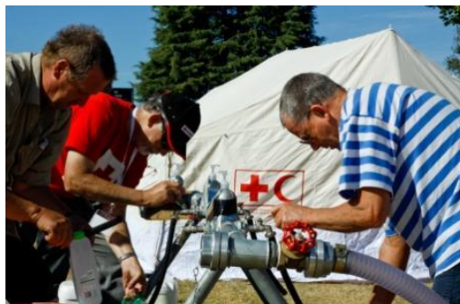
Ensuring safe water supply to the people affected by the earthquake in Christchurch, New Zealand. Photo Credit: New Zealand Red Cross.
