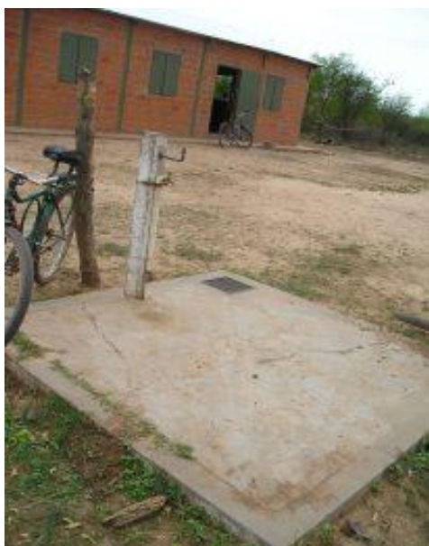
Filtration and water deposits coming from the tajamares in the community of La Preciosa, department of Boquerón.
