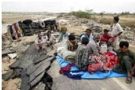
National highway damaged due to floods in Barmer district of Rajasthan Courtesy www.alertnet.org
