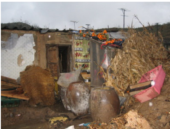
A destroyed home in Ambyon County
