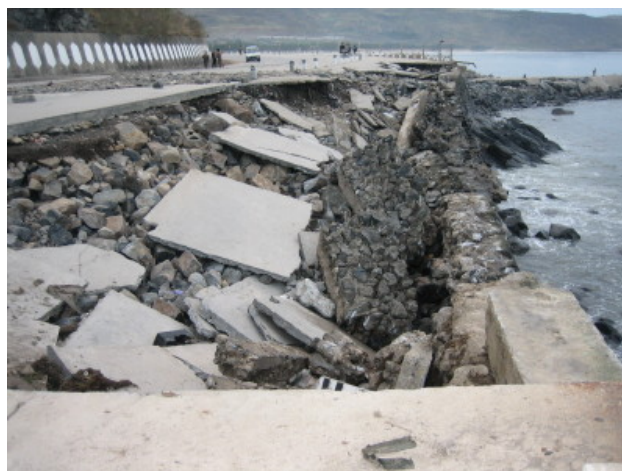
Damage of main road to Tongchon County
