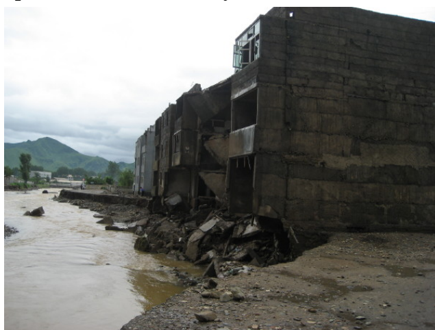
Affected apartment block in Koksan (International Federation/Aug 2007)
