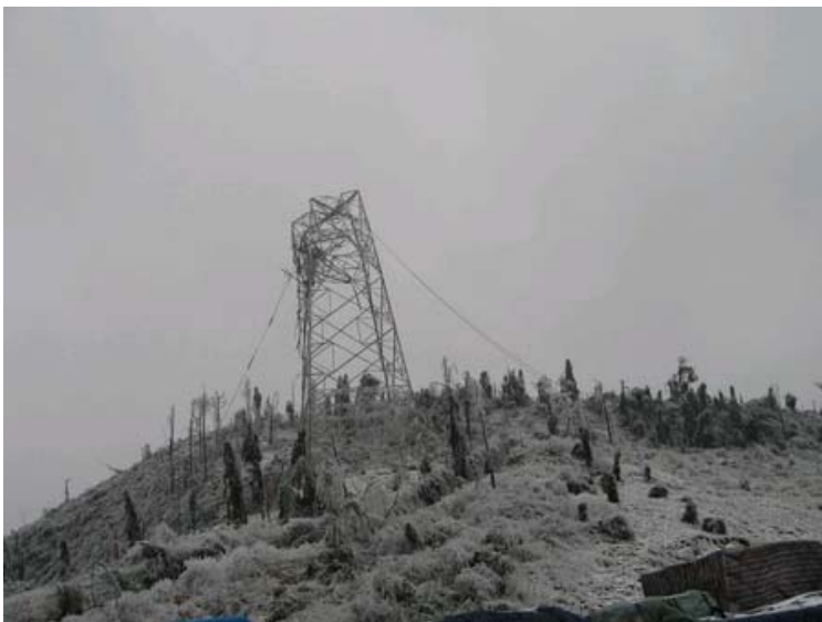
Heavy snow and thick ice on power lines pulled down a power station in Hunan province. Power transmission in Hunan has been badly hit following 20 days of unrelenting snow. Currently, just half of the total power demand is being met in Hunan and the province's 19 plants have 430,000 tons of stored coal. Tragically, to date, 11 electricians have died in the effort to restore power supplies in snow-hit China. RCSC
