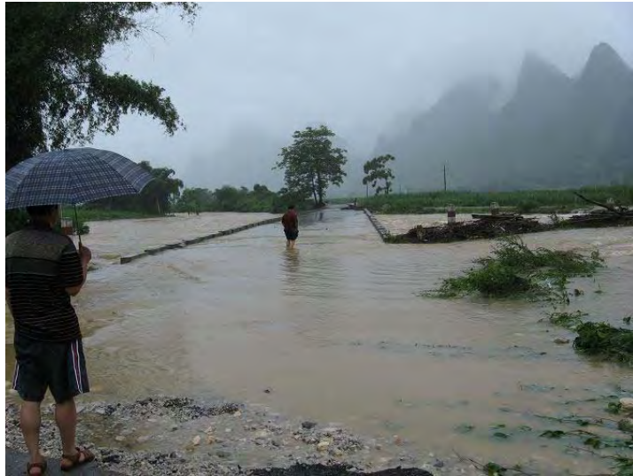
Roads were damaged by the floods in Yizhou Prefecture, Guangxi province. Guangxi branch of the Red Cross Society of China.
