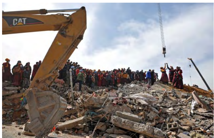
Large excavation machineries reached the quake zone to speed up excavation. More roads and bridges linking Gyegu town with the local airport and other major prefectures were cleared of debris and access resumed, with emergency and relief items are coming fast for the victims. Photo: Xinhua News Agency.
