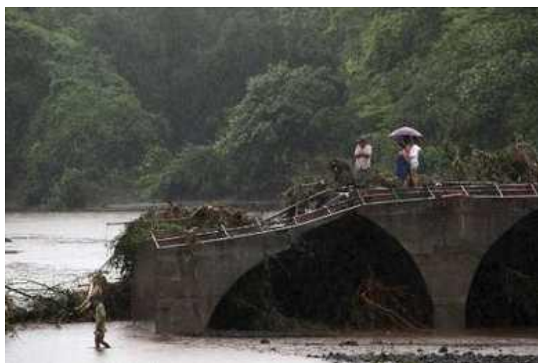
Farmers look at a bridge damaged by heavy rain at Quezalguaque town, some 135 km west of the capital Managua, 21 May 2010. Thousands of people have been affected the flooding caused by heavy rain on the Pacific coast of Nicaragua. Source: REUTERS/Oswaldo Rivas
