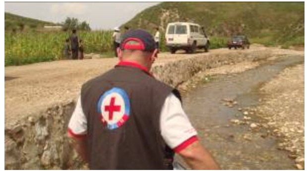
This reinforced river bank in Jongchuk Farm, Songchon county, South Pyongan province is an effective intervention to mitigate the possible effects of floods and mudflows.
