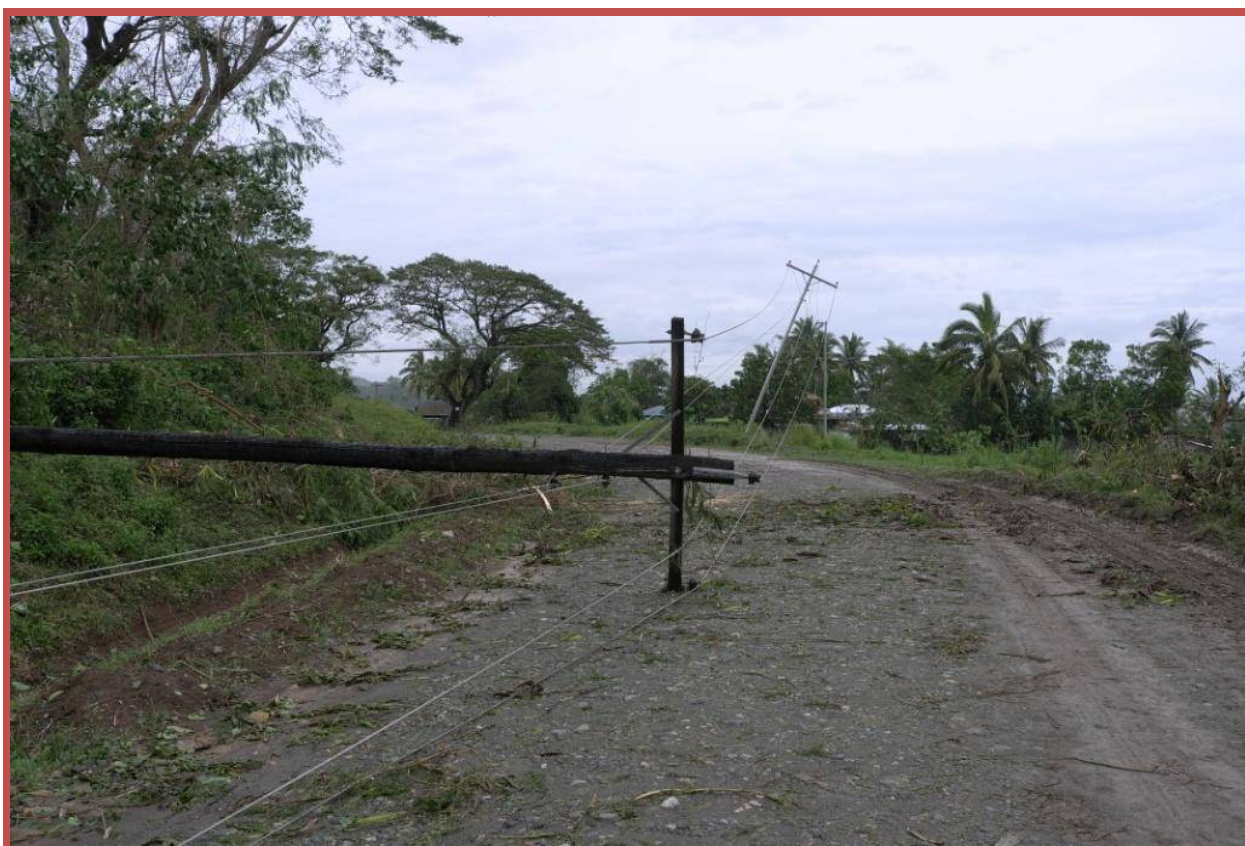
Typhoon Megi smashed into the Philippines with powerful force. Winds toppled electrical posts – causing power outages – and uprooted trees. Fallen electrical posts meant a dark night for residents of Kalinga. Photo: Hajime Matsunaga/IFRC
