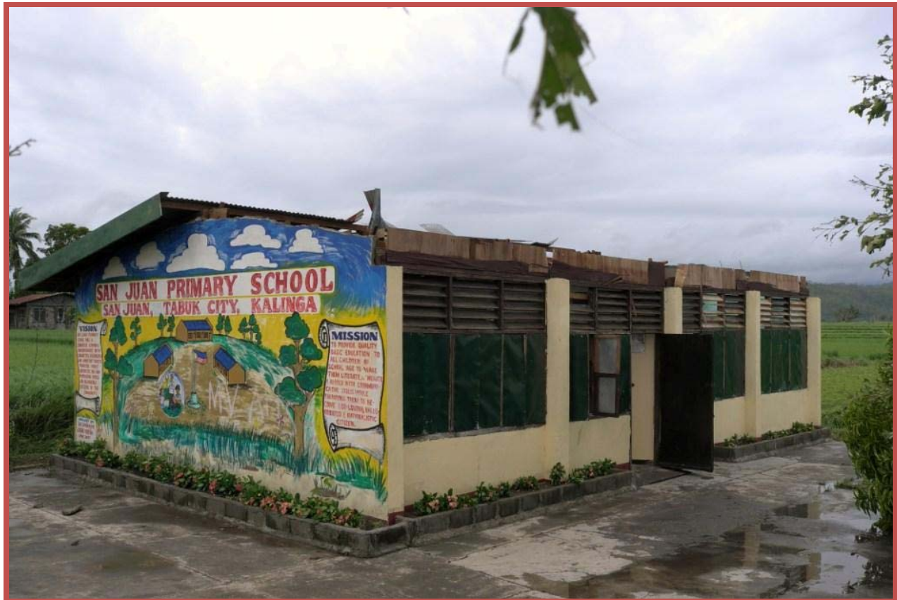
This elementary school suffered considerable damage, with its roof blow off by the strong winds Photo: Hajime Matsunaga/IFRC
