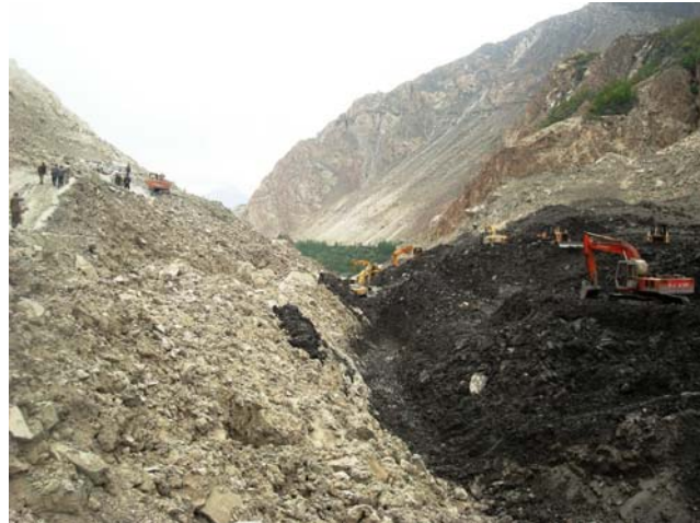
Federal Works Organization working to excavate the spill way. Photo: Local website.
