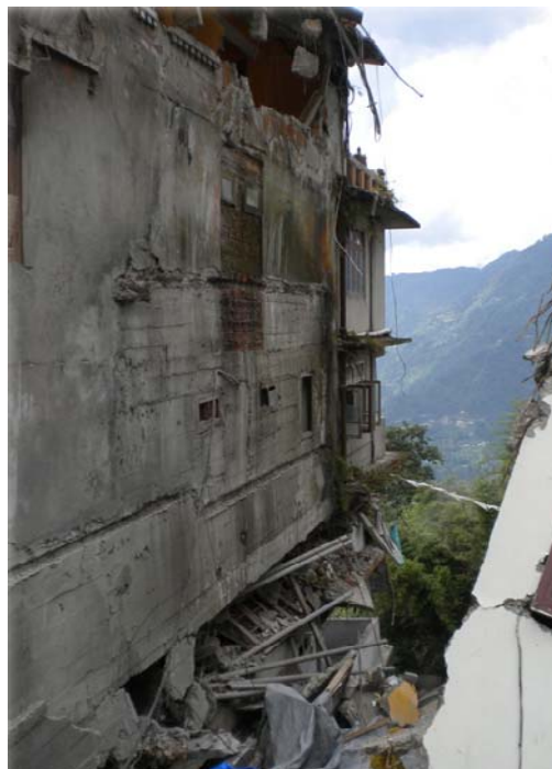
The destruction/ damage caused to infrastructure and building structures by earthquake in sikkim. Photo: IRCS NDRT member.
