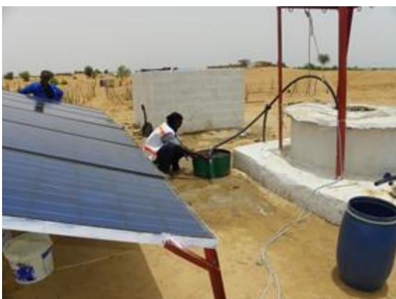
Functional water points rehabilitated with solar powered pumps. Photo: IFRC/MRCS
