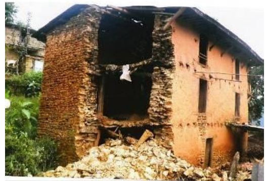
One of the damaged houses in Sindhupalchowk. Photo: NRCS.
