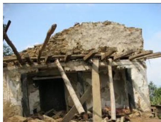
Another damaged house found in Panchthar district. Photo: NRCS.
