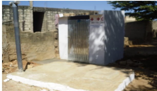
A fully rebuilt latrine in the district of Cité Lamy/ Photo: SRC
