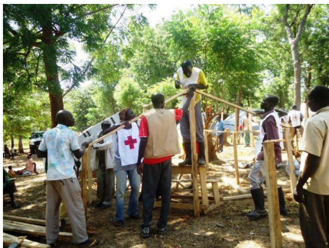
Cameroon Red Cross volunteers are constructing emergency shelters in Northern Cameroon, with the full participation of people who have been displaced by unprecedented floods. / Photo by Cameroon Red Cross
