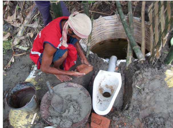
Construction of toilet for the flood affected people. Photo: Indian red Cross Society.
