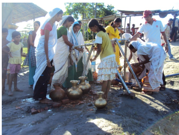
Water purification unit installed in Salmara providing purified water. Photo: Indian Red Cross Society
