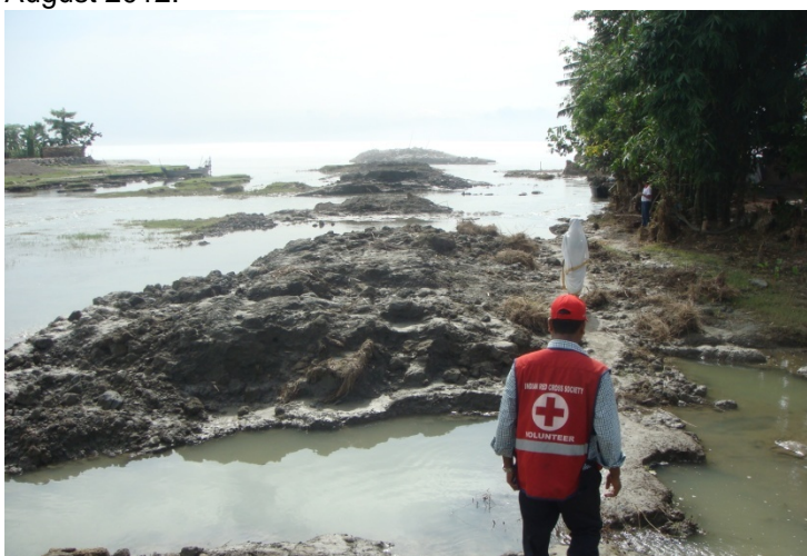
Gushing flood water swept away embankment in Majuli Island which resulted in inundation of villages. Photo: IRCS/IFRC joint assessment team.
