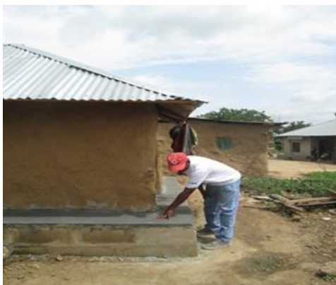
Raised cement foundations are built around houses in Odogwu, Kogi as a simple measure to protect them from future flooding. Photo: IFRC/NRCS
