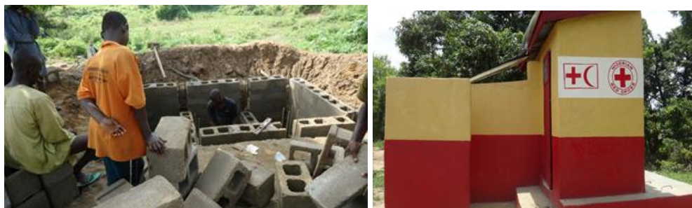
In Ozahi, Kogi state, 7 latrines have been constructed (6 household and 1 institutional). Photo: IFRC/NRCS
