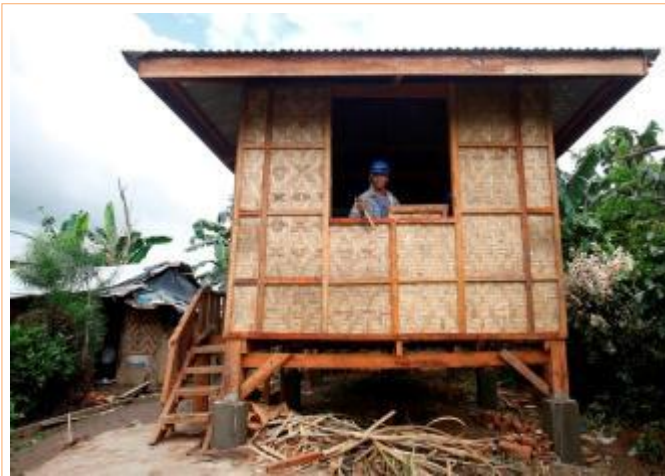
A worker builds the wooden model at Barangay Macopa in Monkayo, Compostela Valley. The all-wooden structure mainly targets families who lived in inner barangays whose houses were destroyed where transport of heavy (concrete) materials would be difficult. Photo: Cheryl Gaglac/IFRC.
