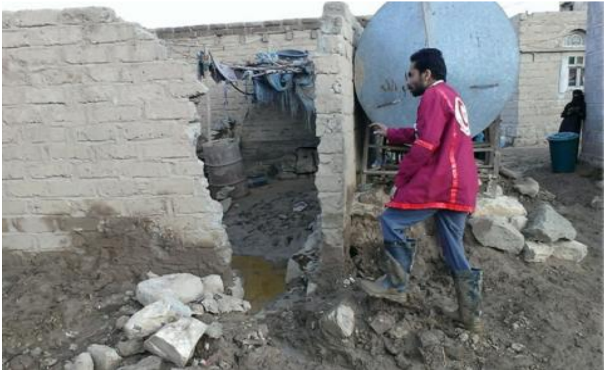
A YRCS Amran branch volunteer assessing damage caused by the heavy rainfall. Source:YRCS
