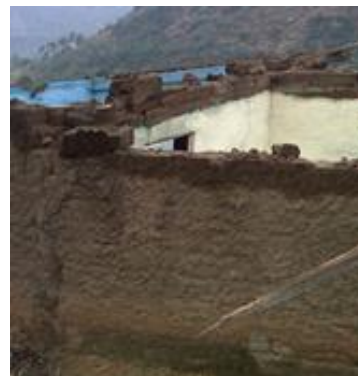
Many houses were unroofed in Leribe and Maseru. Photo by Lesotho Red Cross
