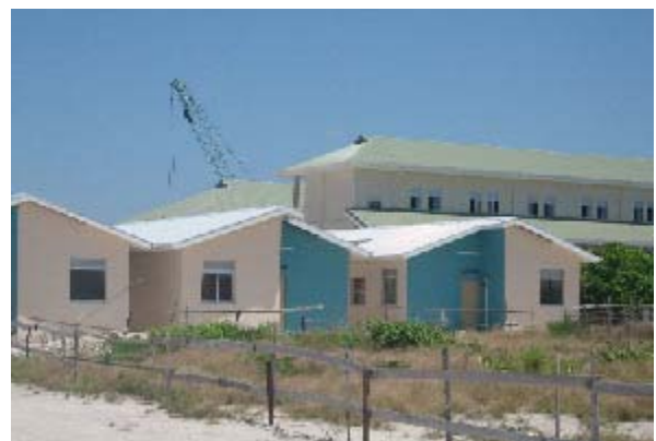
Considerable progress has been made on Dhuvaafaru; the remaining construction works will be completed before the end of this year.
