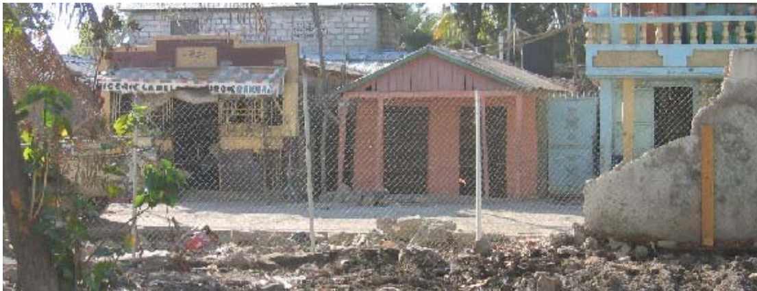
A large piece of La Providence's perimeter wall was totally destroyed by flood.
