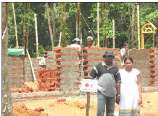
Mr. and Mrs. Sandun de Silva stand outside the construction of their new home in Beruwela, southwest Sri Lanka. Belgium Red Cross is funding reconstruction of some 500 houses along the damaged coastline.
