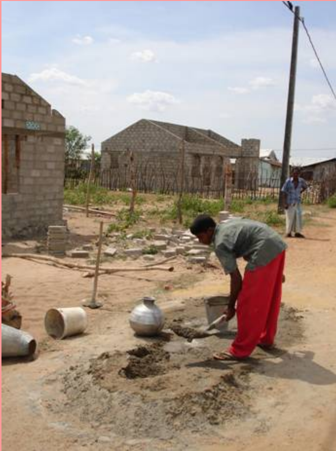
Reconstructing his own home: Construction is finally underway in the Vakharai region north of Batticaloa, where recent fighting forced tsunami survivors again to seek temporary shelter. On this site in Mankerny, 98 families will be completing the reconstruction of their own homes with the help of top-up grants from the CRRP, funded on this site by the Australian Red Cross. International Federation/Vibeke Greni.
